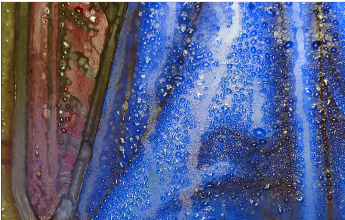
Figure 15. Condensation on the internal glass surface.
