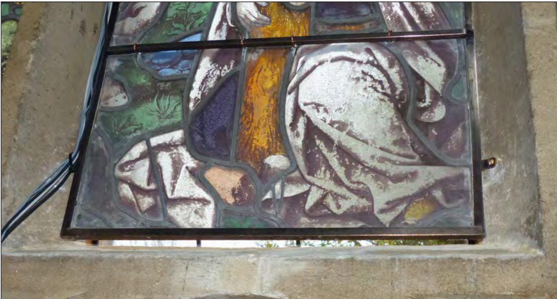
Figures 7, 8. Ventilation openings at the top and bottom of a recently installed internally vented system at the Vyne, Berkshire.
