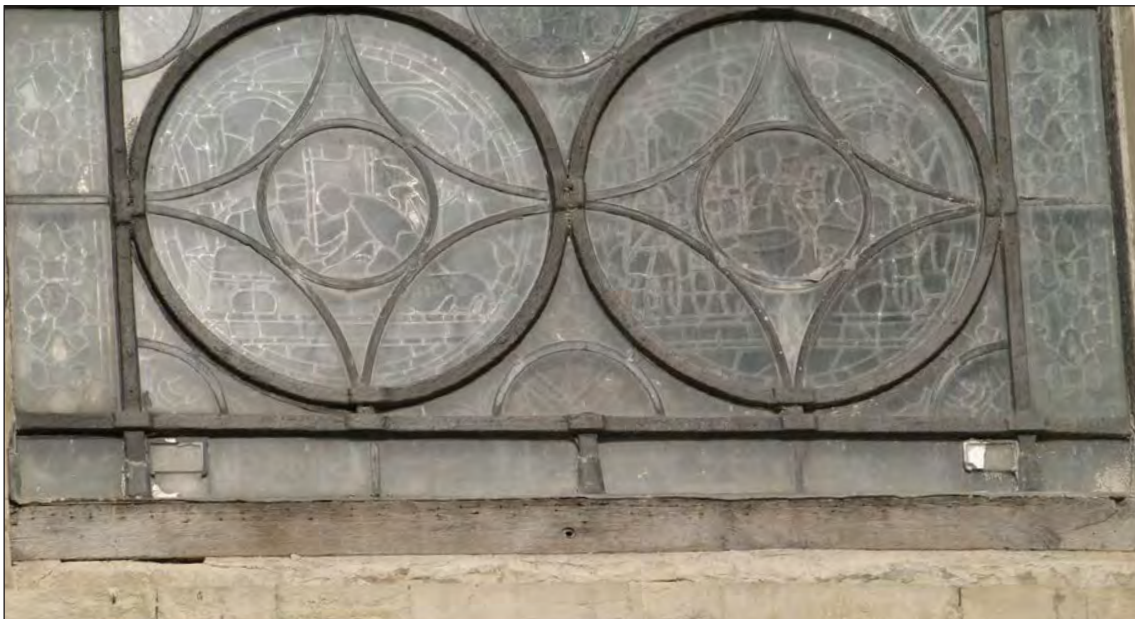
Figure 24. Ventilation openings at the bottom of an externally vented system installed in 1979 at Canterbury Cathedral.
