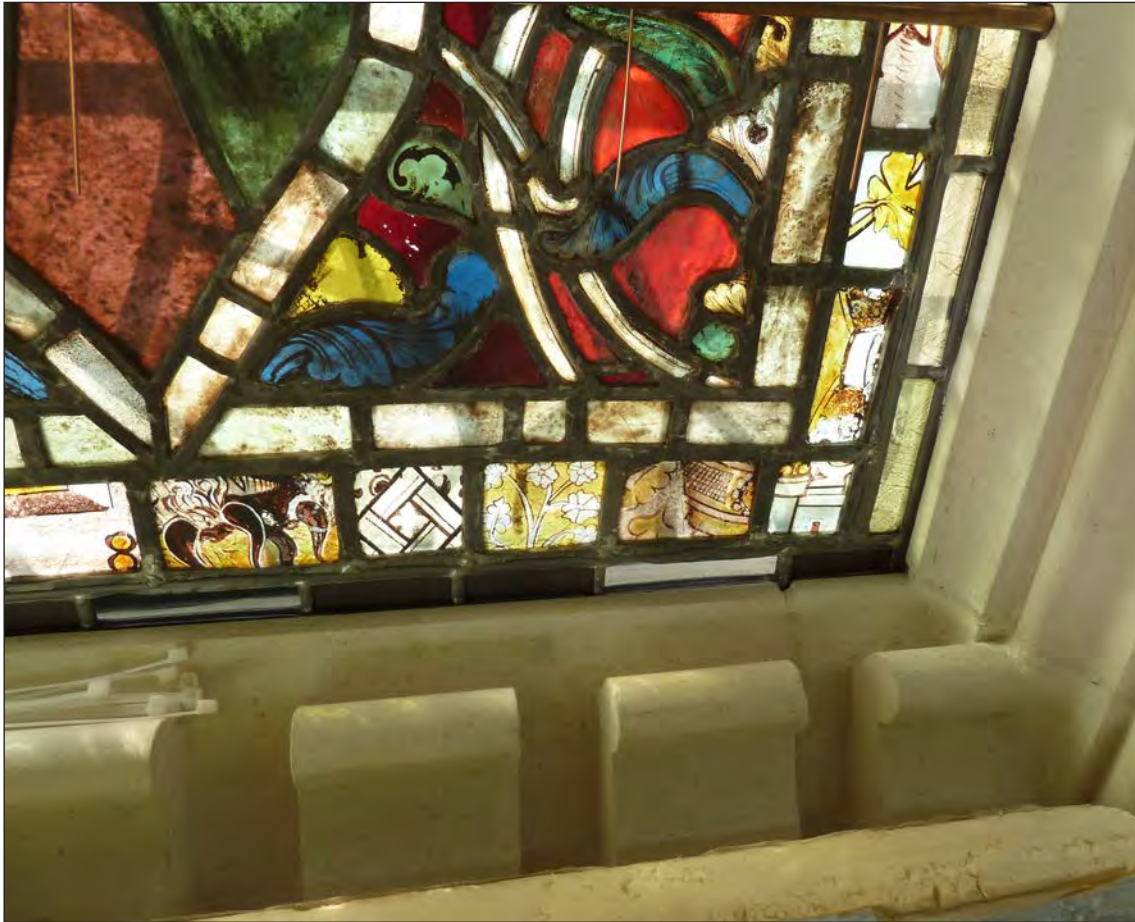
Figure 29. Ventilation openings at the base of the Great South Window at Canterbury Cathedral.
