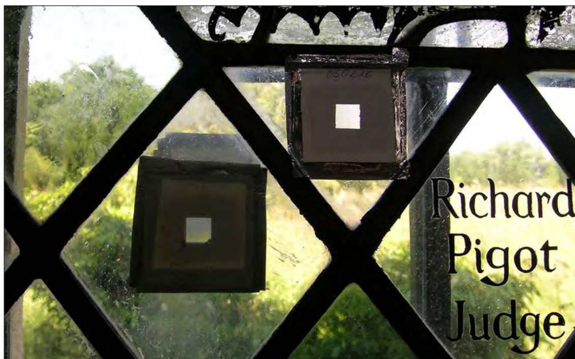
Figure 38. Glass sensors in place on the internal and external faces of the glazing at Holy Trinity Church, Long Melford.
