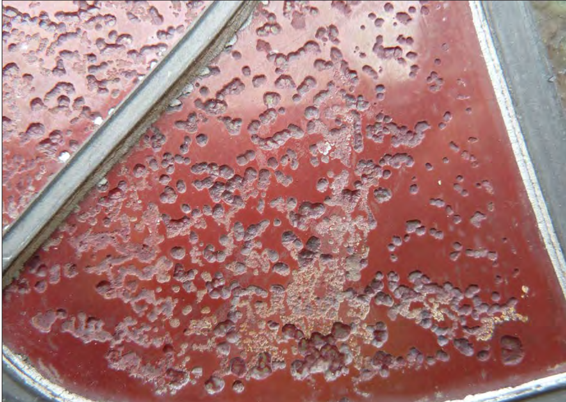
Figure 2. Closer inspection reveals corrosion pits have damaged the red glass layer.
