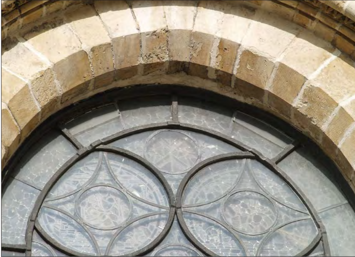
Figure 25. Ventilation openings at the top of an externally vented system installed in 1979 at Canterbury Cathedral.
