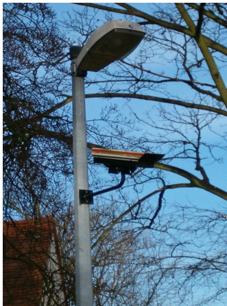
External CCTV camera on lamp post.
